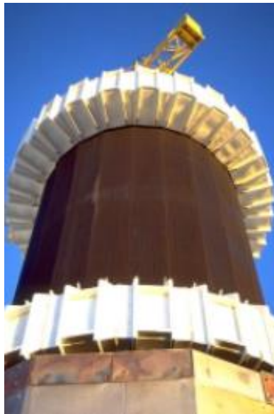
Figure 17. Solar Two receiver. Figure extracted from [47].
